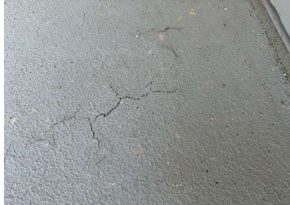
Figure E6 (33685): Drill 1" hole through finish BELOW crack in upper-level deck waterproofing. Inspection will be provided via endoscope.
