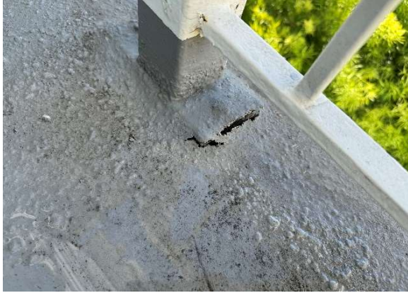
Figure E1 (24416): Remove deck topping to fully expose gaurd rail post, post base, base connection (screw/bolt). Extend removal in 12" each direction to expose top of plywood deck.
