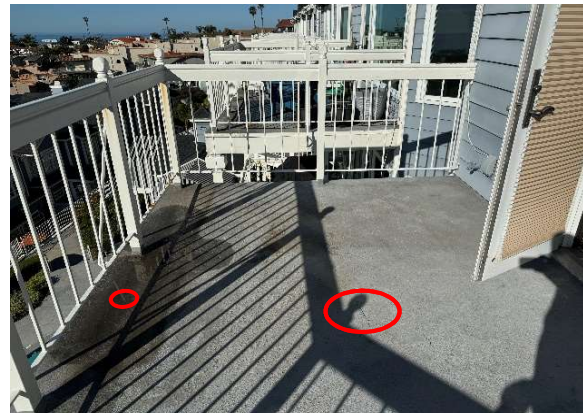
Figure E4 (24436): Drill 1" hole through wood soffit finish BELOW two noted areas in the upper deck where: water is ponding and at large crack in waterproofing. Inspection will be provided via endoscope.
