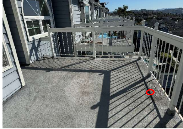
Figure E2 (24424): Drill 1" hole through wood soffit finish BELOW this area of the upper deck where water is ponding. Inspection will be provided via endoscope.
