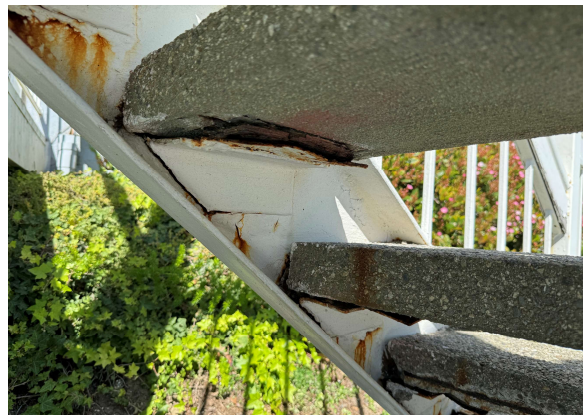
Figure 12: Severely rusted stair tread ledger angles.
