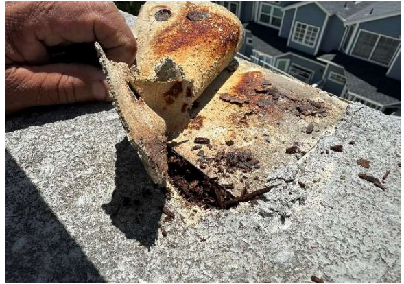
Figure 6: Rotted plywood below ponding area.
