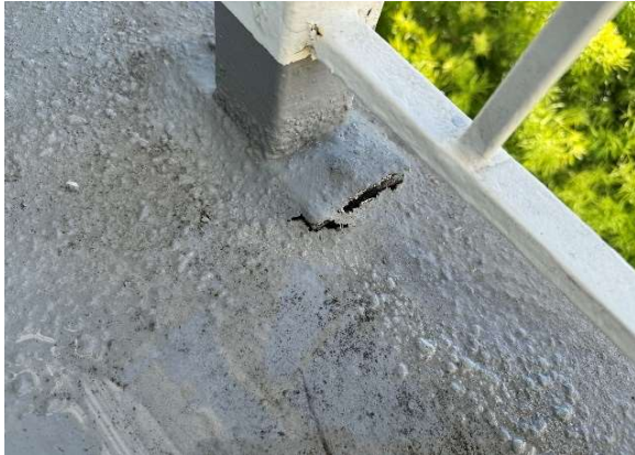
Figure 1: Typical decking with damage at guardrail post.
