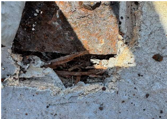
Figure 3: Severely rusted baseplate and rotten plywood photographed during intrusive inspection.
