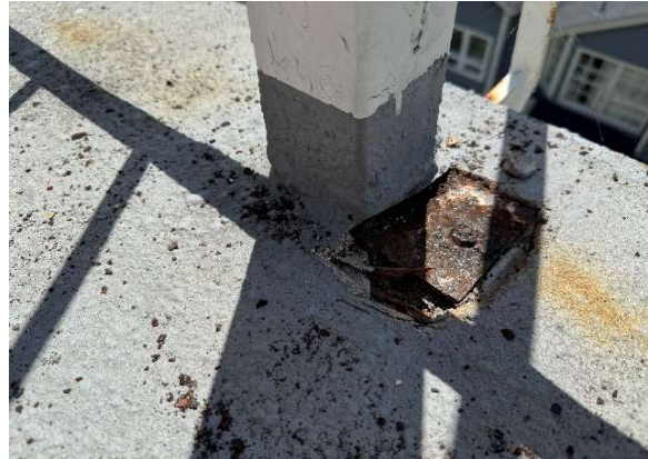
Figure 2: Severely rusted baseplate and rotten plywood photographed during intrusive inspection.
