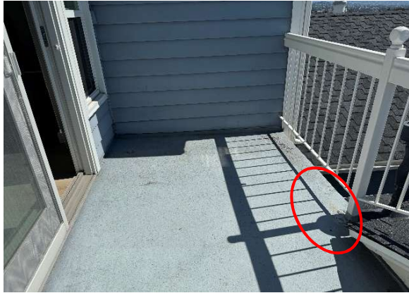
Figure 9: Granada upper (Master) balconies at typical area of water damage at guardrail post. Note this is a low point in the deck and a point of drainage.
