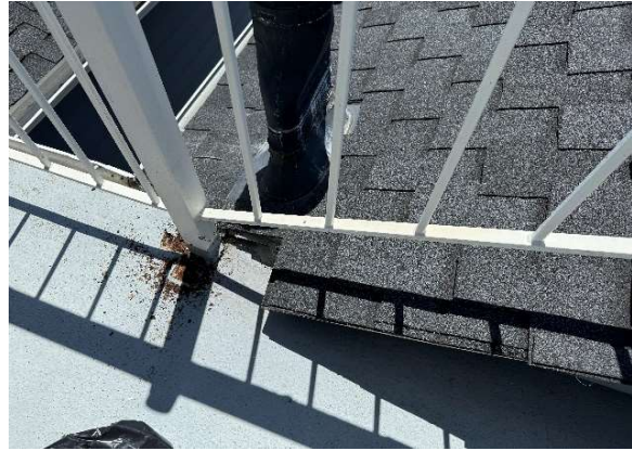
Figure 10: Baseplate exposed to show severe rust damage and damage to structure below.
