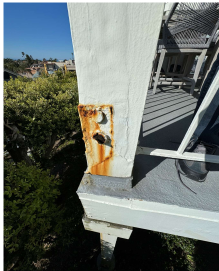
Figure 4: Severely rusted post-to-post strap.
