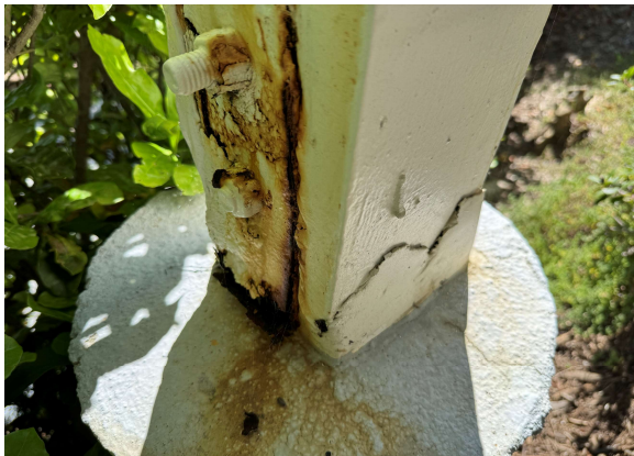
Figure 7: Typical post base with severe rust.
